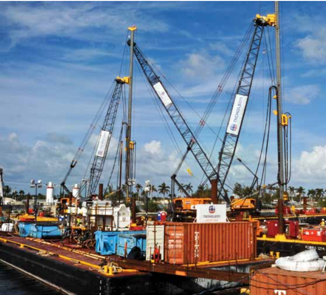
Offshore grouting operations require the contractor to mobilize and remobilize each week to keep cruise ship traffic flowing uninterrupted.
