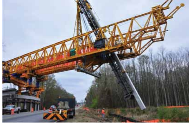
Custom tilting pile driving led by Bermingham Foundation Solutions at work for Top-Down Bridge Construction of Washington, N.C.
