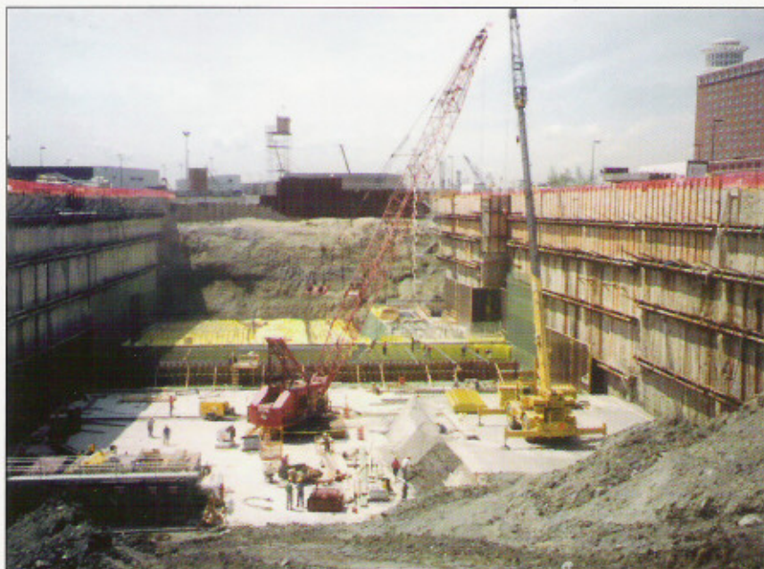
70 ft deep excavation for Logan Airport approach to the Ted Williams Tunnel – C07A1 Bird Island Flats.
